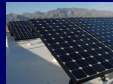
Photovoltaic (PV) panel
