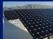
Photovoltaic (PV) panel
