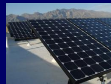
Photovoltaic (PV) panel
