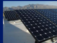
Photovoltaic (PV) panel
