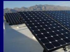
Photovoltaic (PV) panel
