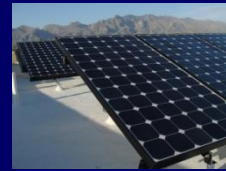
Photovoltaic (PV) panel
