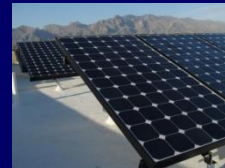
Photovoltaic (PV) panel
